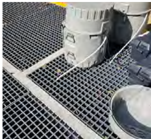
ISCO at effluent.
