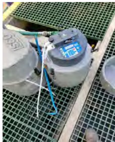
ISCO at Effluent
