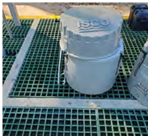
ISCO at effluent
