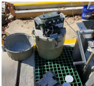
ISCO at effluent.
