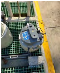
ISCO at Effluent
