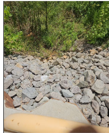
No water flow at outlet
