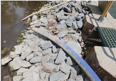
No water flow at inlet
